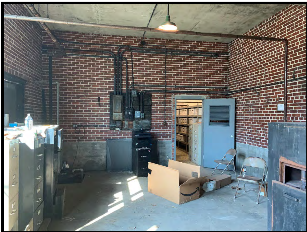
Photograph 22: View of boiler room that leads to file room in western portion of property.
