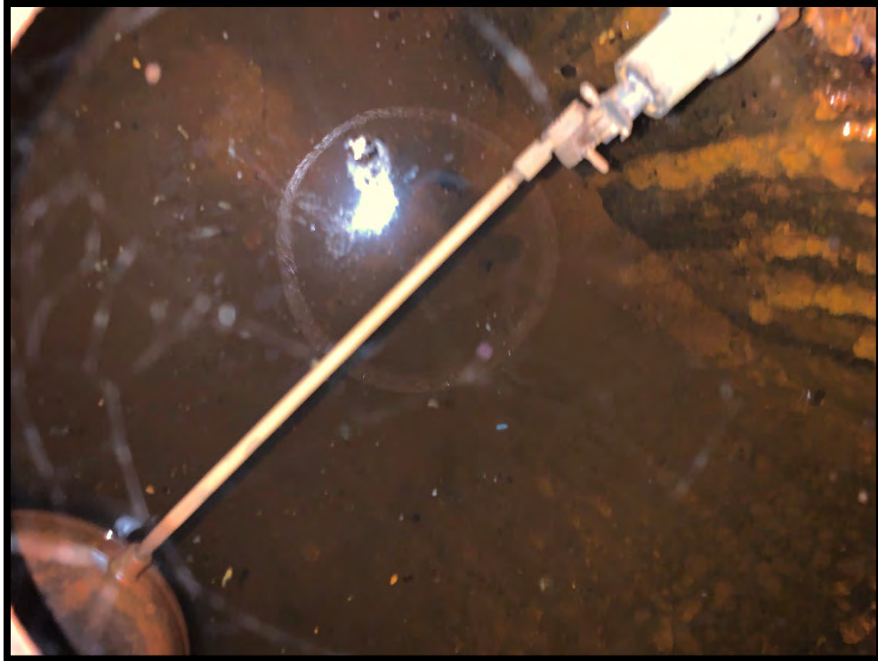
Photograph 21: View of standing liquids inside of storage tank adjacent to boiler (pictured above).
