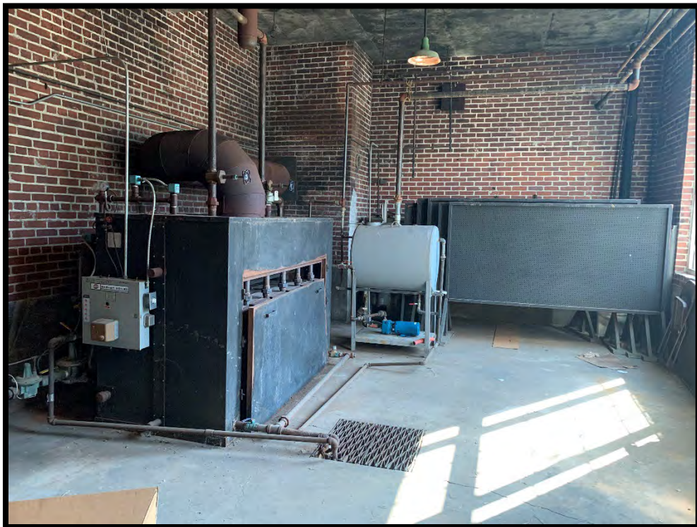
Photograph 20: View of boiler and tank in western portion of building.
