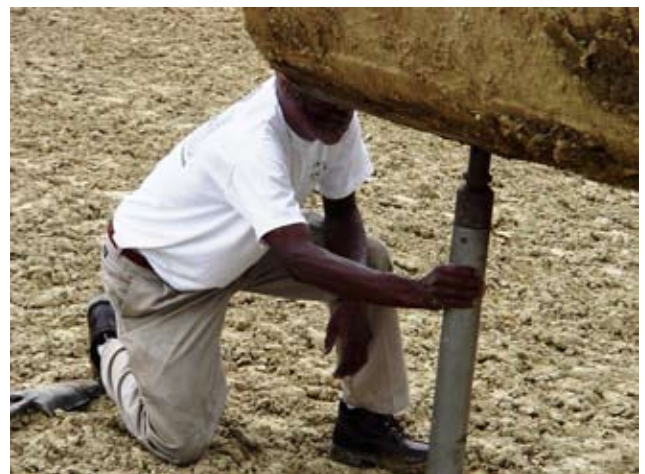
Figure 10D–32 Shelby tube sample being obtained with backhoe bucket used to force tube into clay liner (Photo credit Jody Kraenzel, NRCS, NE)
