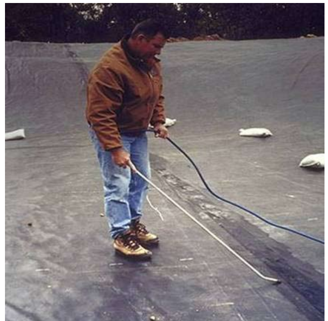
Figure 10E-19 Air lance test
