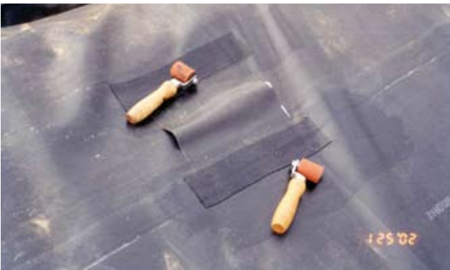
Figure 10E-29 Covered liner vent
